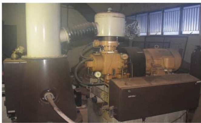
Liquid Nitrogen Plant
